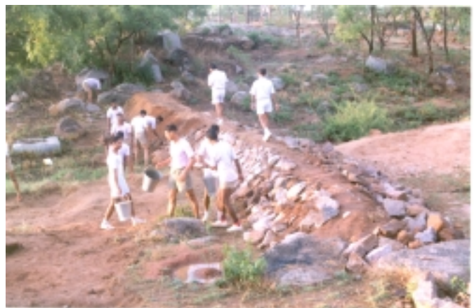
Staff and Trainees of NISA building a bund under the Rain Water Harvesting Scheme.
